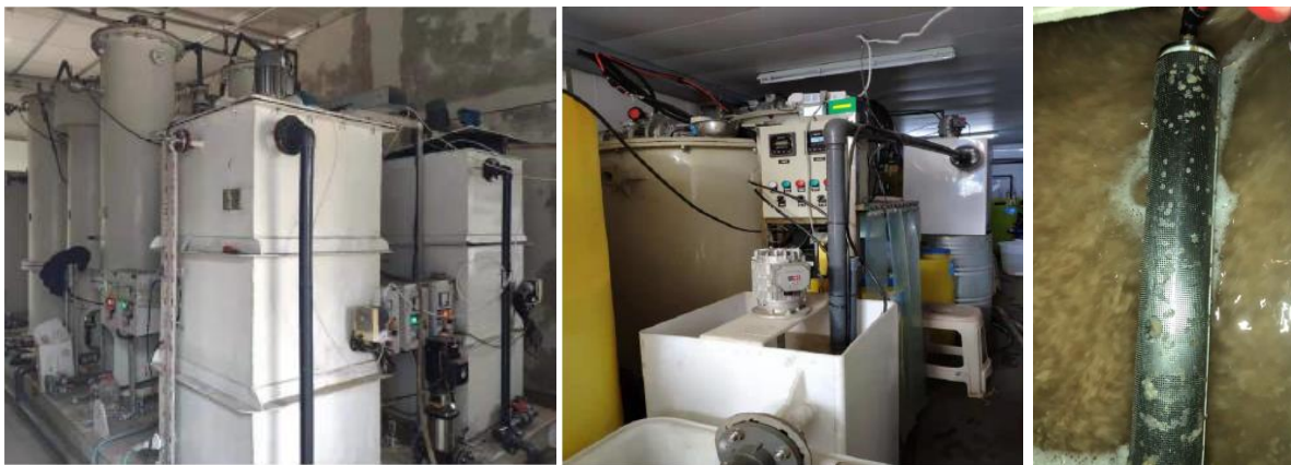
Figure 3. Photo of the Pilot Plant Equipment, CIF ® (left), BIOCLENS ® Reactors (middle), Self-Cleaning Screen (right)
