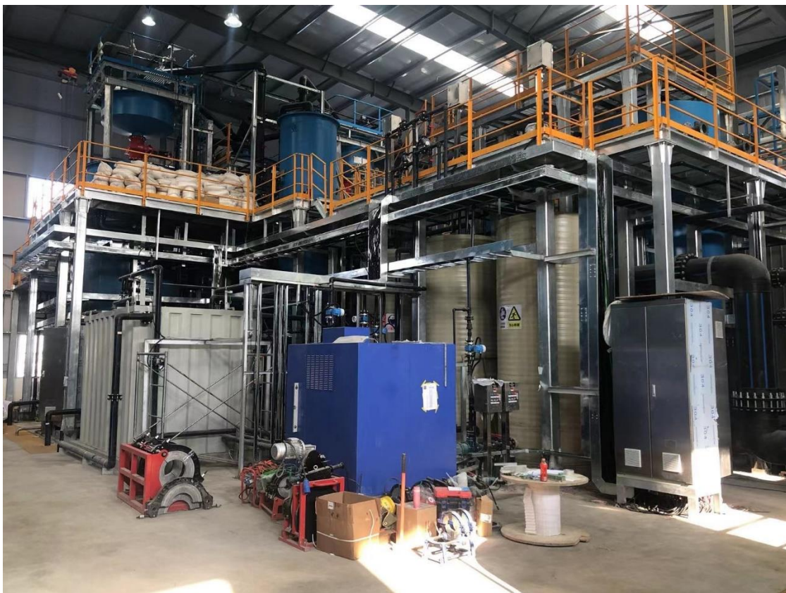
Figure 6. Photo of the BIONEX Nitrate Removal Plant in Ordos, China
