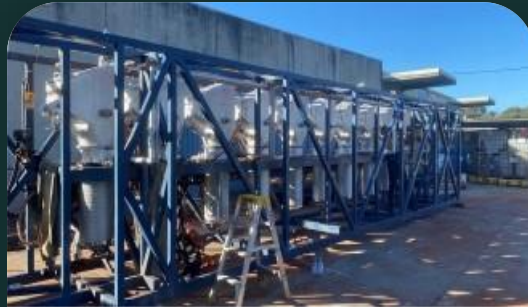
Lithium cDLE® Pilot Commissioning
