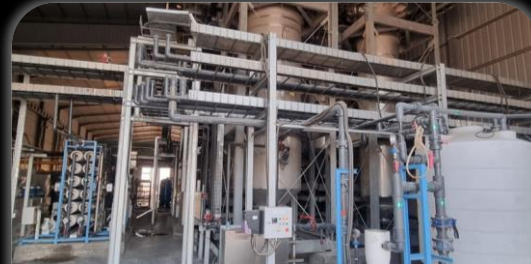
MENA HIROX® Water Recycle Practical Completion
