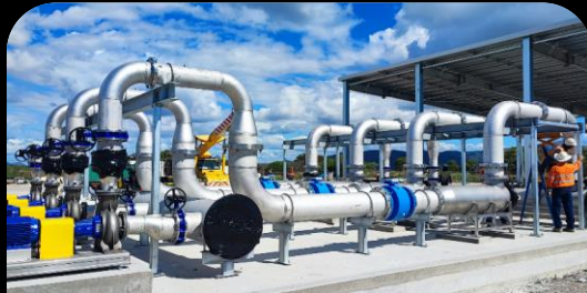
Townsville UV Water Recycle Installation
