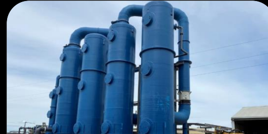
NSW EVAPX® Brine Recycle Commissioning
